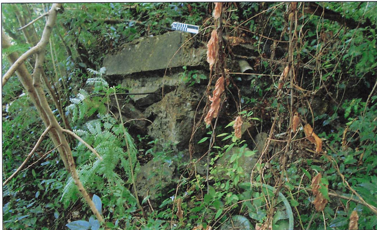
Figure 12: Lot 142-3-3 View east of concrete with rebar, rocks and PVC pipe near northeast corner of lot (photo: J. Farrugia 2/15/2023).
