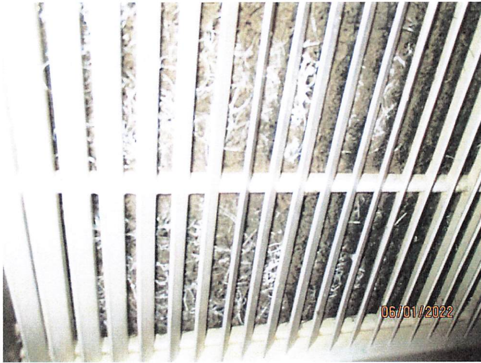
2 ND FLOOR VACANT UNIT NO. 202; CENTRALIZE AIR-CON EAXHAUST LOTS OF MOLDS
