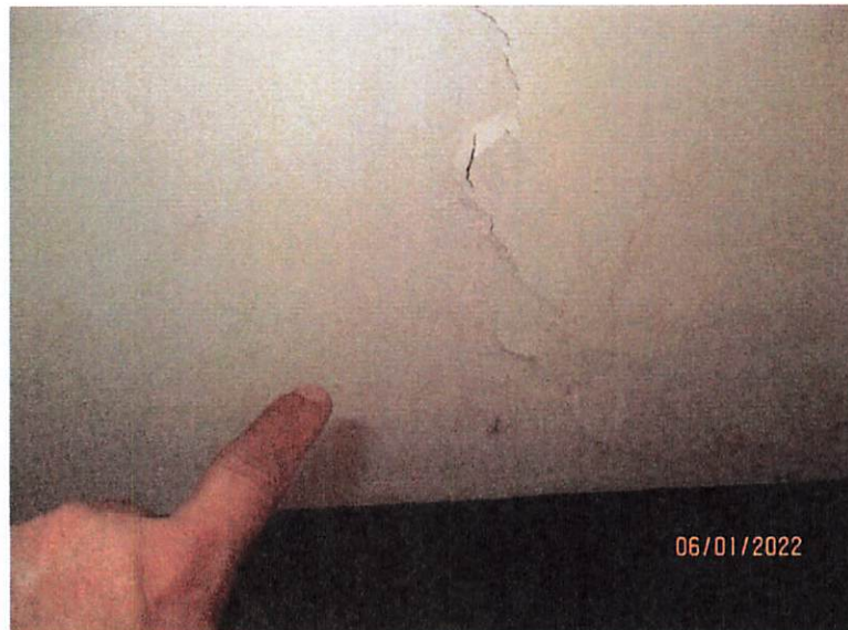
3 RD FLOOR UNIT #3 W/ 2 BEDROOM; BEDROOM #2 CRCK ON THE WALL
