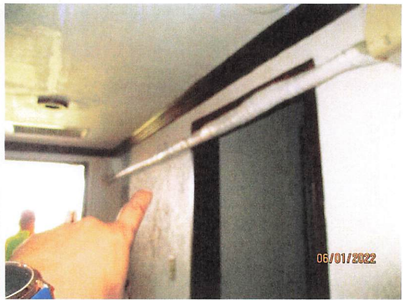
HALLWAY AIRCON CONDENSER PIPE NOT IN PROPER LOCATION
