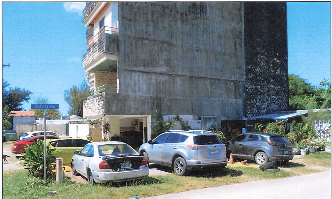
Figure 3: Lot 010 D 12 View northwest from corner of Alahai Avenue and Alus Street showing east elevation (photo: J. Farrugia 1/31/2023).
