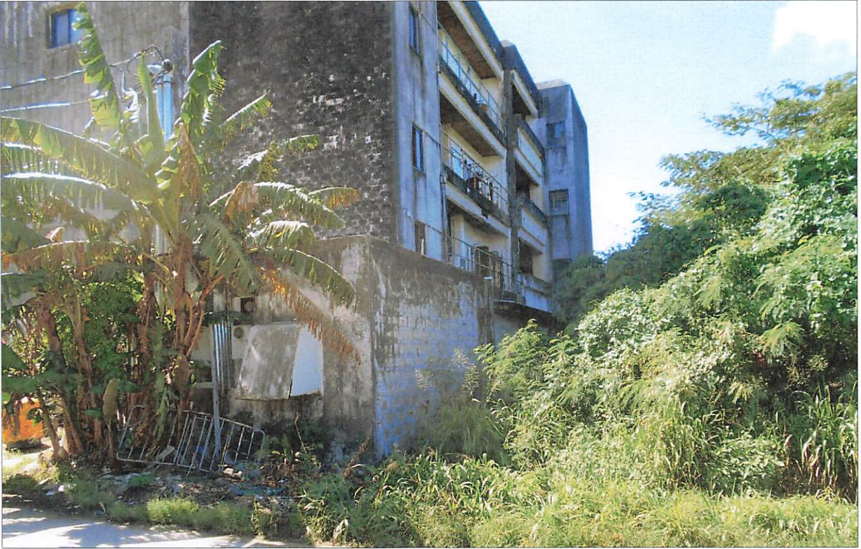
Figure 4: Lot 010 D 12 View west of northeast corner of building (photo: J. Farrugia 1/31/2023).
