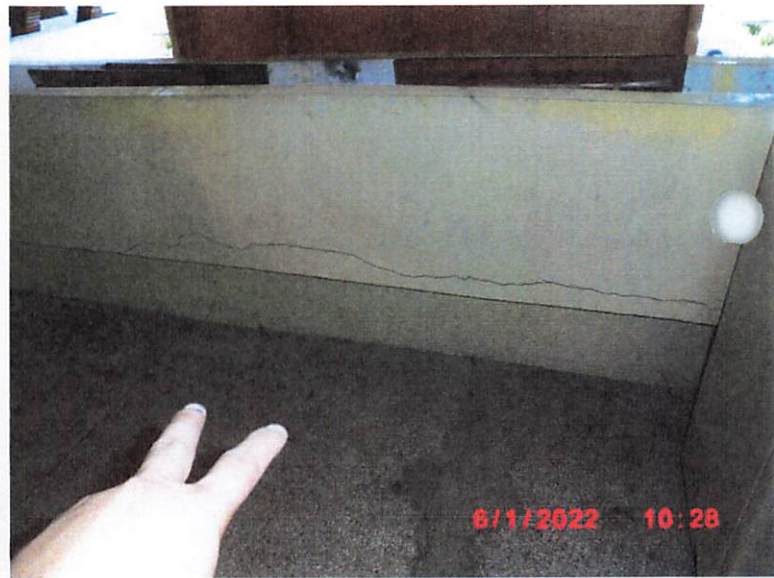
2 ND FLOOR PLANT BOX WALL HAS BIG CRACK
