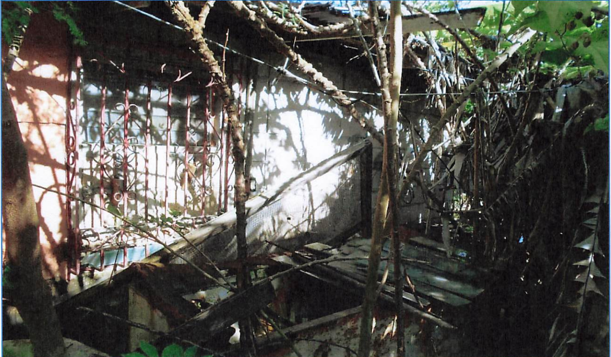
Figure 9: Lot 012 I 05 View north of northeast corner of structure (photo: J. Farrugia 2/23/2023).
