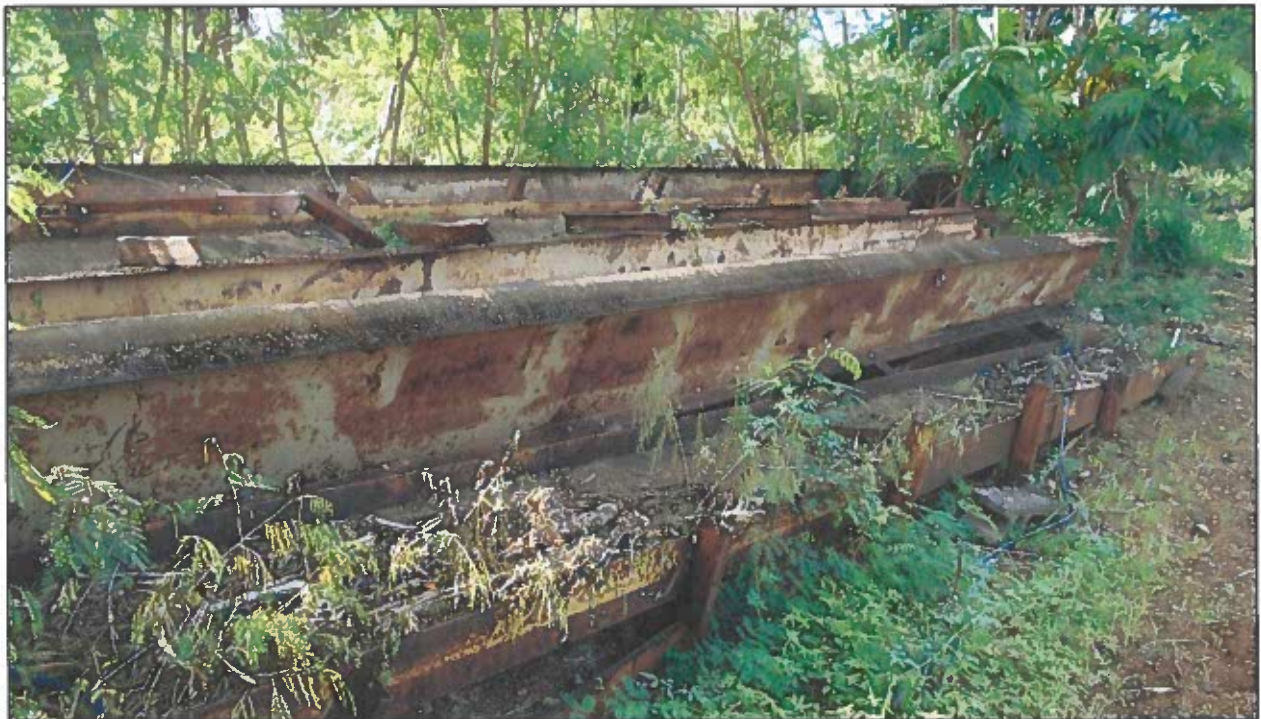
Figure 11: View south of steel I-beams next to entrance road (photo: J. Farrugia 1/24/2023).
