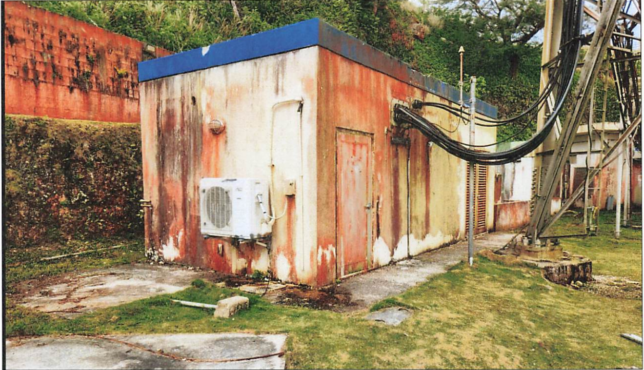
Figure 11: View west of east corner of Building 3 with western leg of tower on right side of photo (photo: D. Perzinski, 6/15/23).
