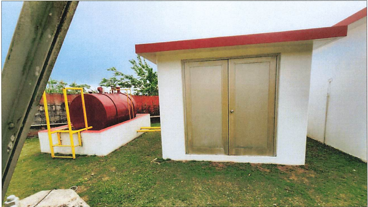
Figure 13: View southwest of northeast elevation of Building 5 and tank (photo: D. Perzinski, 6/15/23).
