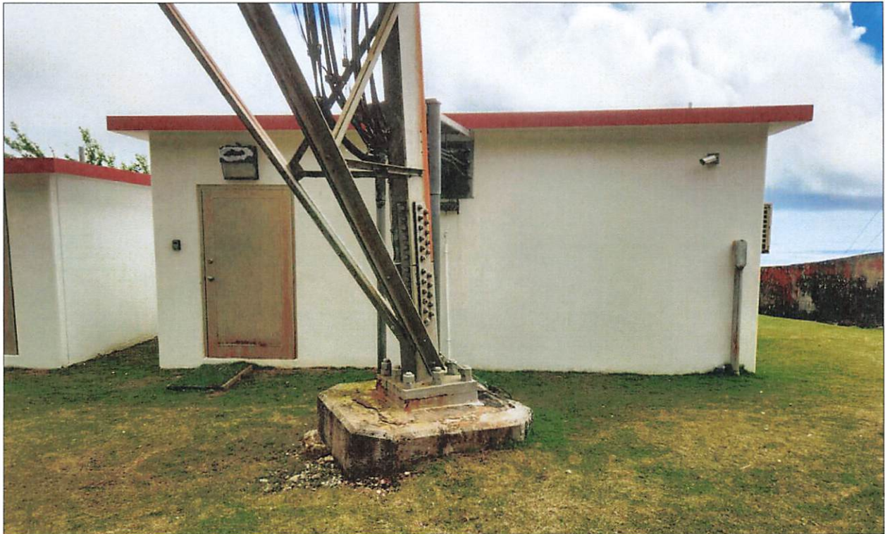
Figure 12: View northeast of southwest elevation of Building 4 and southeaster leg of tower (photo: D. Perzinski, 6/15/23).
