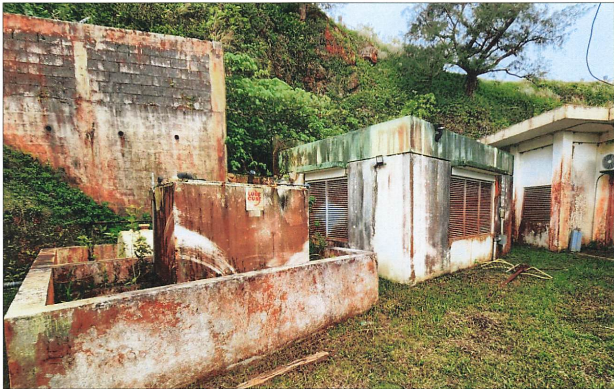
Figure 10: View west of east corner of Building 2 and fuel tank (photo: D. Perzinski, 6/15/23).
