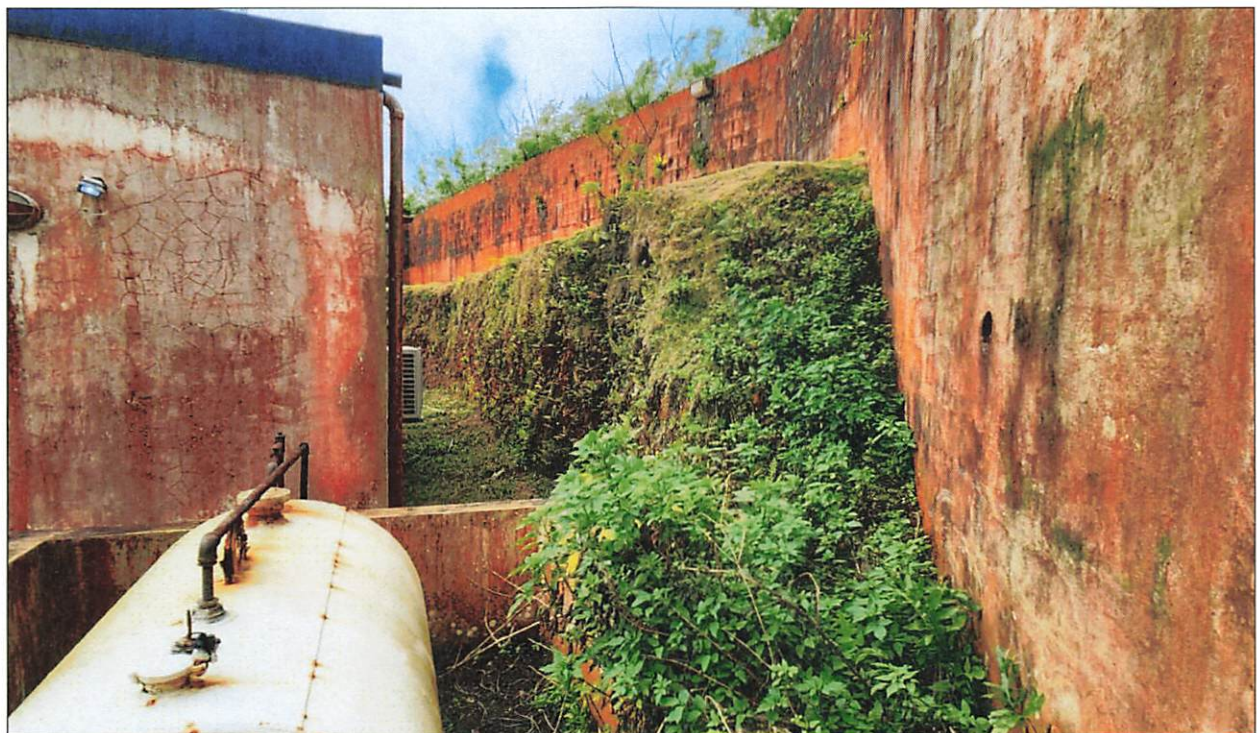
Figure 7: View southeast of bedrock cut and wall on southern end of tower compound (photo: D. Perzinski, 6/15/23).
